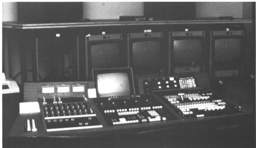
Fig. 4. View of stations in the edit room, showing color monitors and speakers in the background. In the foreground, left to right, are: audio switcher buttons; audio console and meters; control panel and monochrome display monitor; video switcher panel and picture monitor assignment panel.
